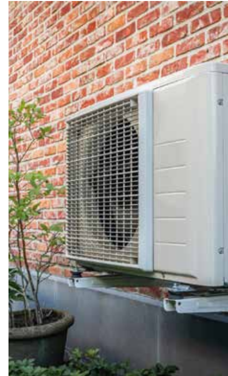
Photo: Heat Pump
